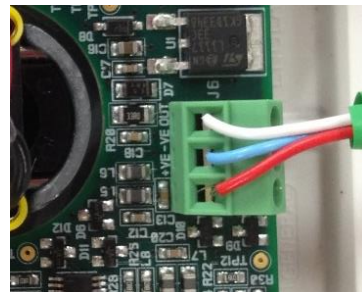
Figure 4 - Alert Management Unit wiring.
